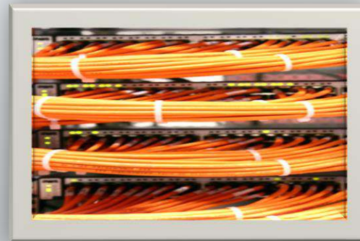
Cable tie Data Centre
